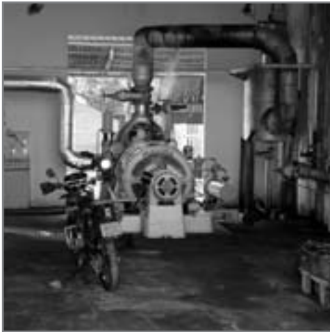
Steam under high pressure passes through the turbine, which again is connected to the generator
