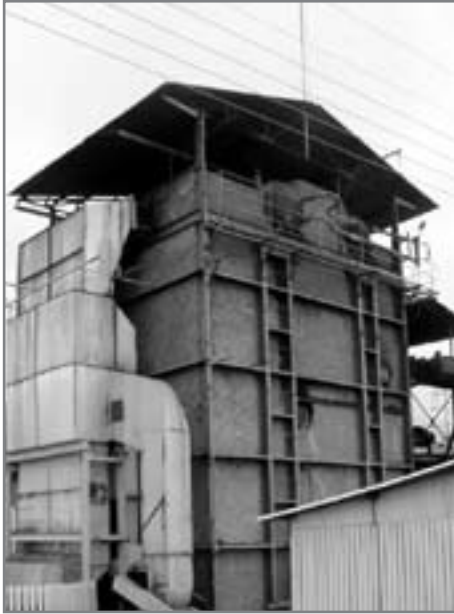
The 1 MW power plant transforms biomass to electricity
